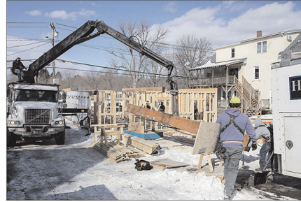
A crew frames the first floor of a multifamily complex in Westbrook, which amended its zoning regulations last year to allow for denser development downtown. "We as a region have a housing shortage," Mayor Michael Foley said. City planners say land-use restrictions, stringent zoning laws and pushback from neighbors are complicating efforts to make the region more livable.
